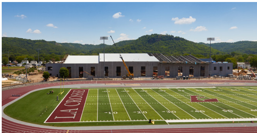
A view of the fieldhouse project from the bleachers of Roger Harring Stadium at Veterans Memorial Field Sports Complex.
