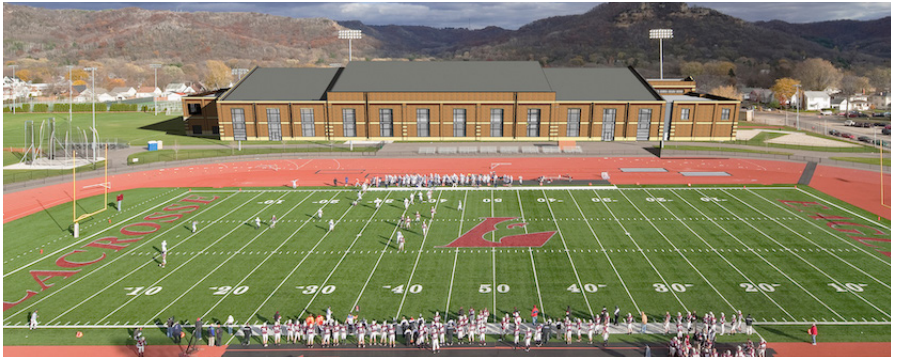
A view of the fieldhouse project from the bleachers of Roger Harring Stadium at Veterans Memorial Field Sports Complex.
