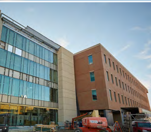
Windows are adorning the north end of the new structure in late November 2017.
